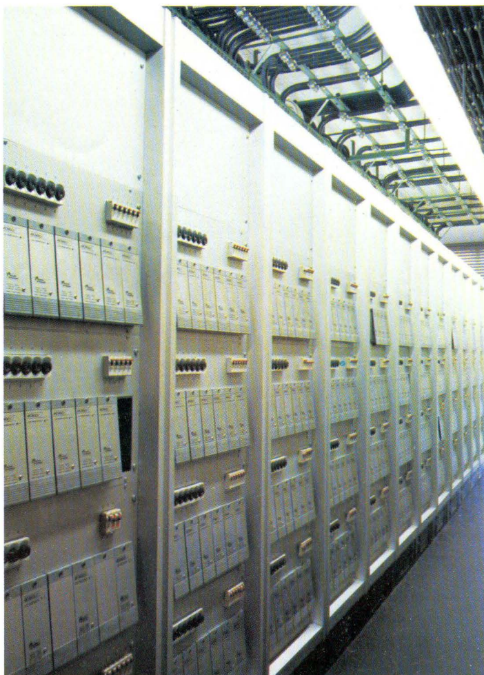
The new MCM (Modular Crate Mounted) dimming system at the Deutsche Oper.
