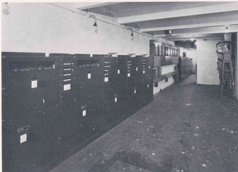
Dimmer room showing STM racks and the vast space vacated by the electro-mechanical banks.
