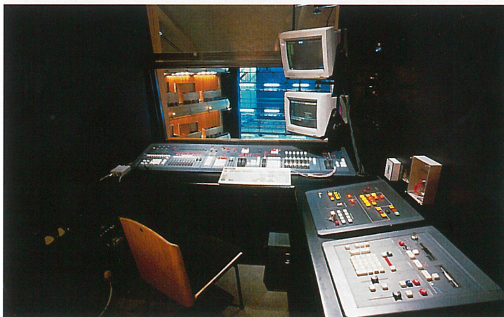
Control room with a Galaxy Nova.
