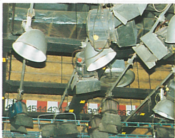
...and the ageing luminaires and steelwork prior to the work commencing.
