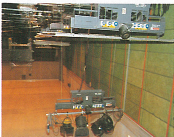
RTM Malaysia's studio in Kuala Lumpur after its transformation by Glantre Engineering and Strand...
