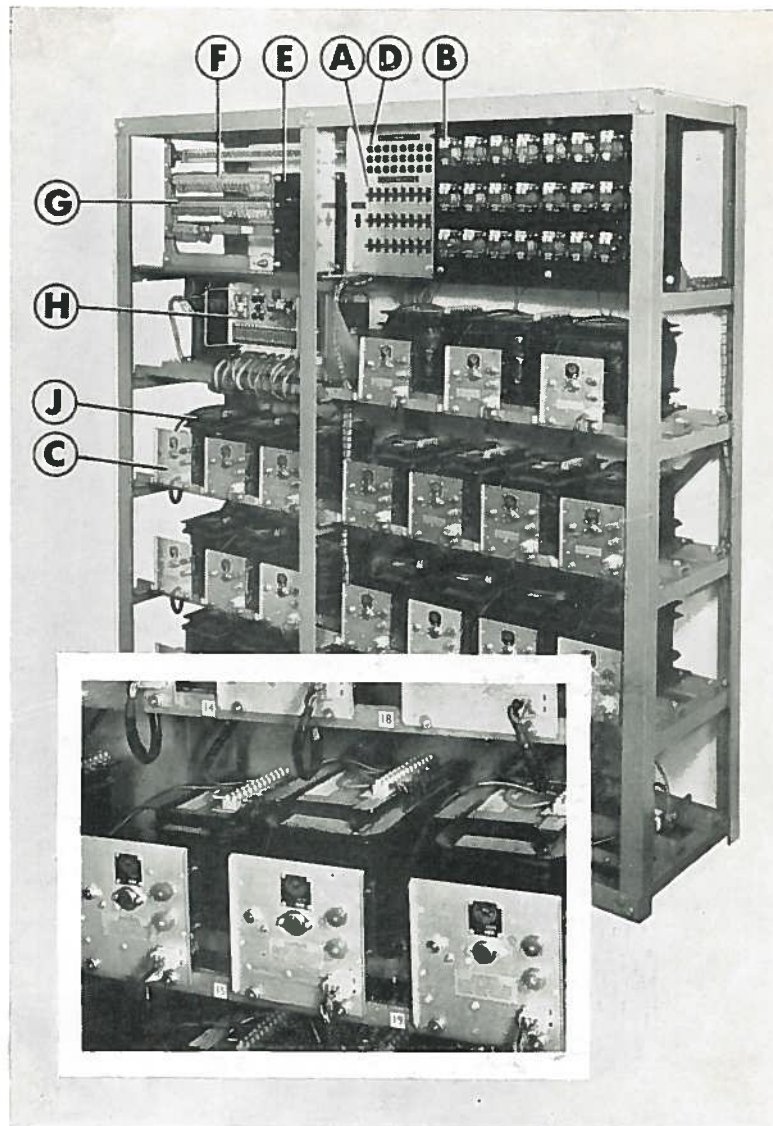
Dimmer Rack for 24 Saturable Reactor Dimmers and their associated control amplifiers. Covers removed.
