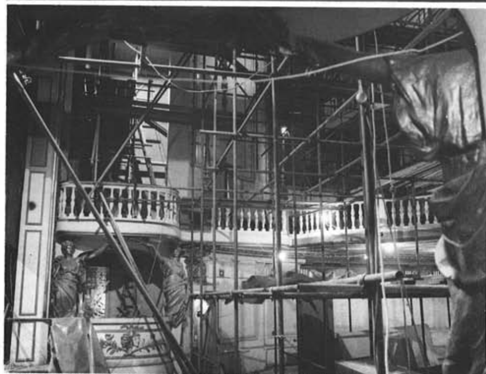
Construction work on the Playhouse began in mid-1986, and the theatre was re-opened in October 1987.
