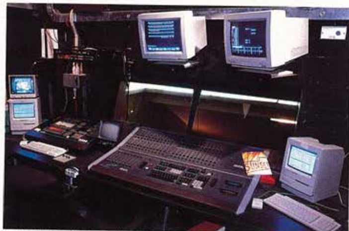
Andrew Bridge's favoured Light Palette 90 and Mini Artisan cheek-by-jowl in the new control room.
