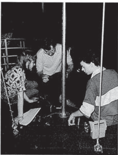
Mike Odam and the electricians get together to deal with a wiring fault.
