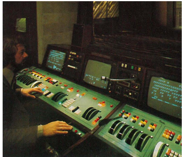
Strand Lightboard, UK National Theatre, 1976
