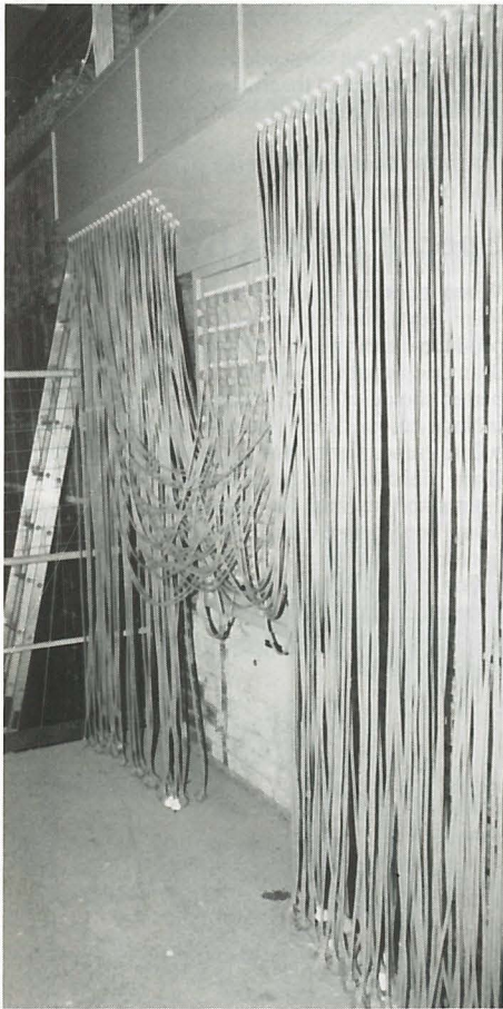
Lighting patch panel – Australian style.
