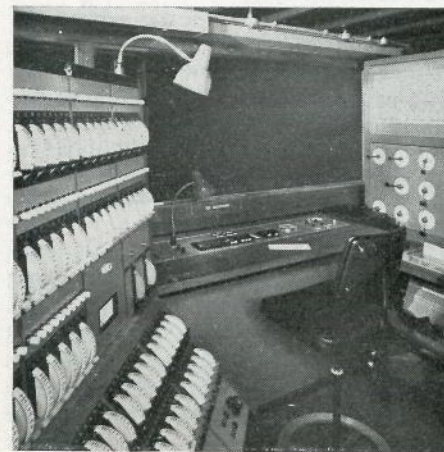
Rank Strand Memocard control system with masters centre under window, channel controls on left and card readers and patching on right.
