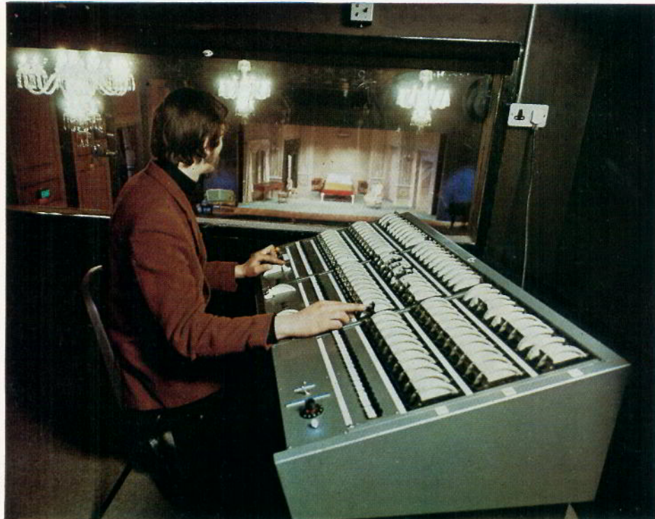
Gate Theatre, Dublin. Operator's view from control room showing S.P.60 3- preset control desk.
