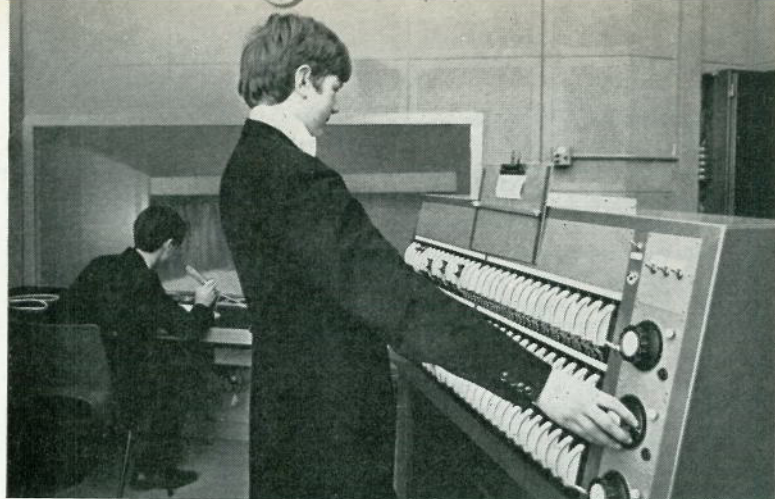
Lighting and sound control room with view of stage through observation window. The Strand control in the picture is a JP60 3-preset but "sound equipment has captured the window space."
