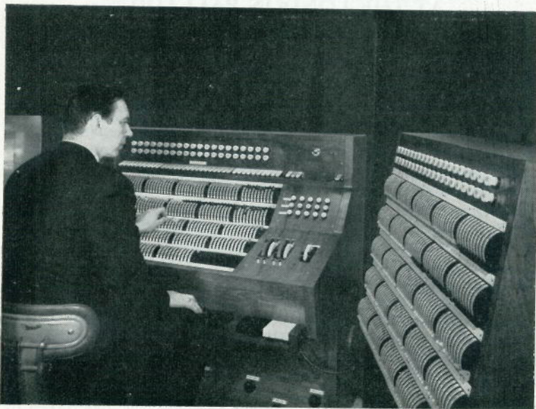
New Lighting Control room at the rear of the Grand Circle, London Palladium. Main 240-channel console on the left and movable preset wing on the right.
