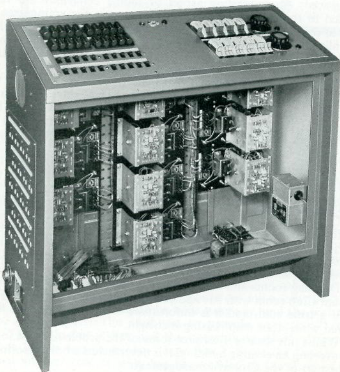
Strand TEN/20 self contained Preset control with cover to dimmer compartment removed.
