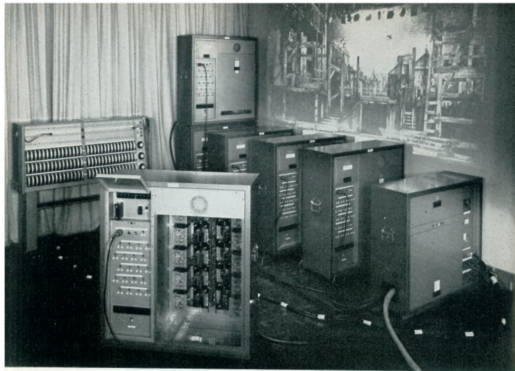
Complete touring lighting control for Oliver! 60-channel 3-preset control, six 10 channel thyristor dimmer units and mains distribution unit.
