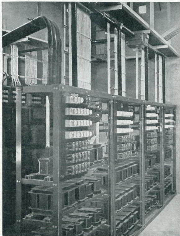
FIG. 5. Reactor choke racks at the Peacock Theatre, Helsinki.
