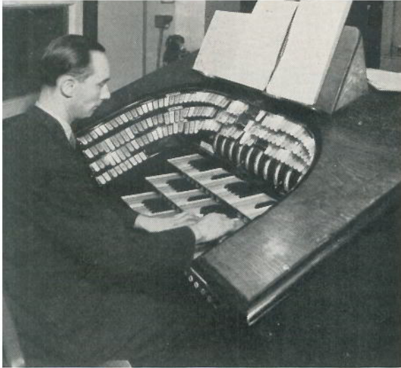
Fig. 1. The Strand Light Console which controls 216 circuits but only measures 4 ft. 9 in. wide by 3 ft. deep by 4 ft. high, including control of all remote colour changes on lanterns. The window through which the operator sees the stage is shown at left
