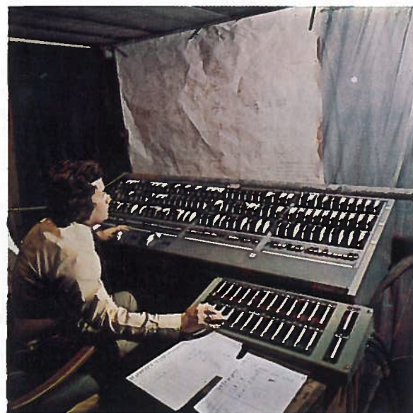
Ice Rink Control Room
