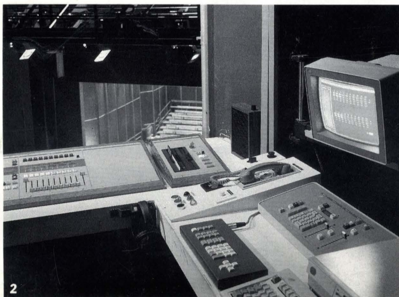
1 PALS installation at the Theatre St. Etienne, Paris. This shot shows part of the F.O.H. rig. The PALS equipment is on Cadenzas, but is available on nearly all our Strand & Quartzcolor units.
