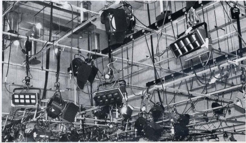
Plenty of Quartzcolor aloft! But note the simple barrel grid. These are still being installed in North America in 1988, simply because T.V. 'over there' has a vast amount of studio space and schedules that demand standing sets. The self climbing hoists and telescopes of intensively used European studios are rare indeed in North America.
