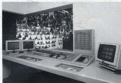
Galaxy II lighting console with memory backup left and PALS control right
