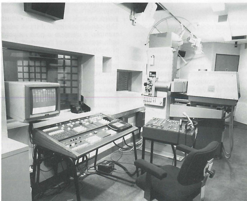
Control Room, Redhill seen from Lighting Desk end. Photo: Dennis Gilbert.
