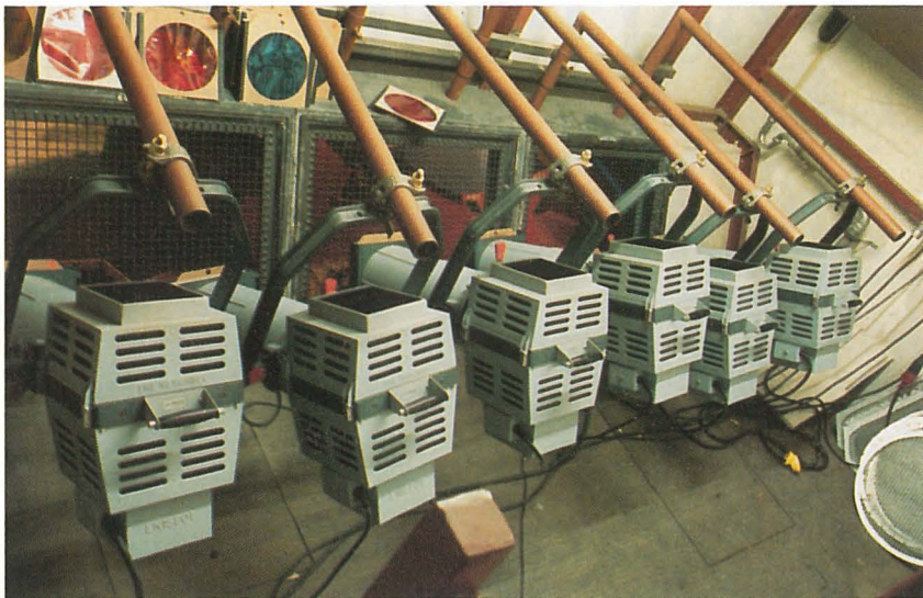
The permanent beam lighting positions of the Deutsches Theatre.
