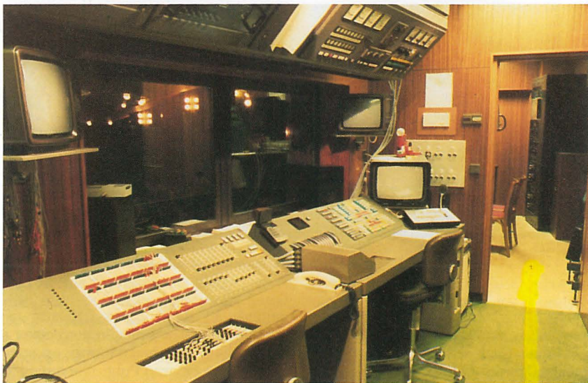
The lighting control room of the Deutsches Theatre contains a Siemens Sitralux B-30 lighting control board and is outfitted with a special pin patch effects program.
