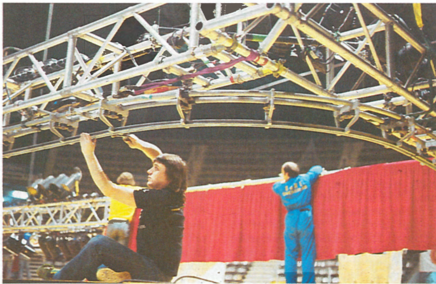
Detail of Loadspan Truss and drape track fitted.
