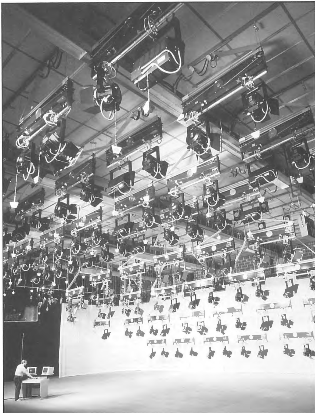
This new television studio in Hannover has probably the world's most sophisticated automated lighting facility. A studio floor control panel allows both lighting levels and positions to be adjusted to a high degree of precision.
