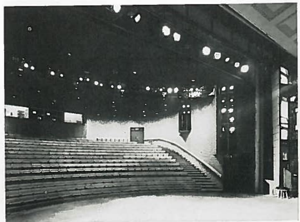
Stage lighting and electrical installation. Thorndike Theatre, Leatherhead.
