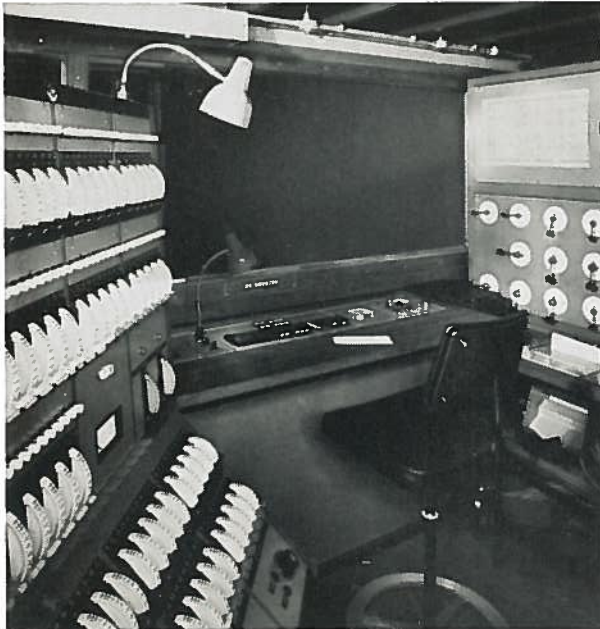
Rank Strand Memocard control system for 100 channels in the Allardyce Nicoll Studio, Birmingham University. Masters are seen centre under window, channel controls on left and card readers and patching controls on right.
