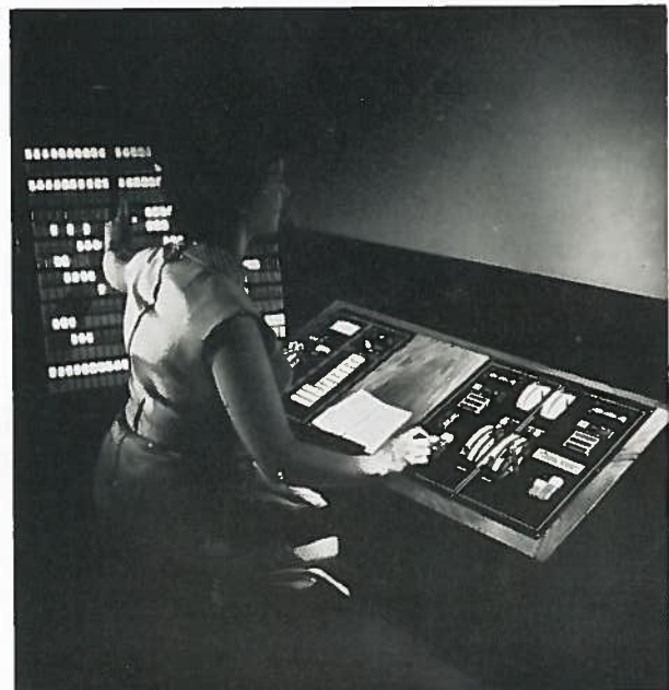
Rank Strand System DDM. Individual rocker tablet controls for 240 channels are on the wing. Dimmer memory controls and numerical selector to break sequence is on the left of the desk and the playback controls on the right.
