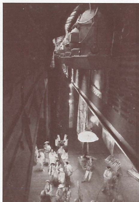
Pattern 76 lanterns fitted with remotely operated colour change at the London Palladium
