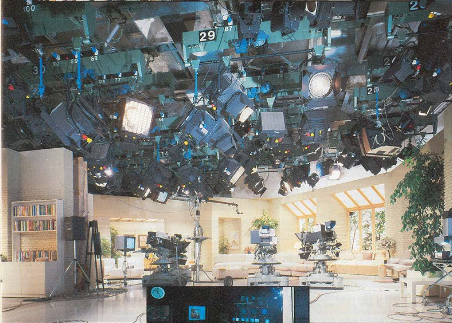
1 Studio A. Hoist detail, showing the Kahouteks on barrel roller trolleys, the Iris 4 cyc lights on pantographs, and the twin cyclorama track on the right.
