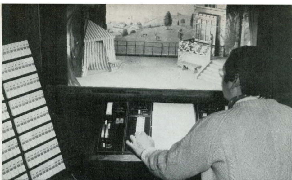
View from new control room before completion of 1972 alterations; system DDM control desk in foreground.
