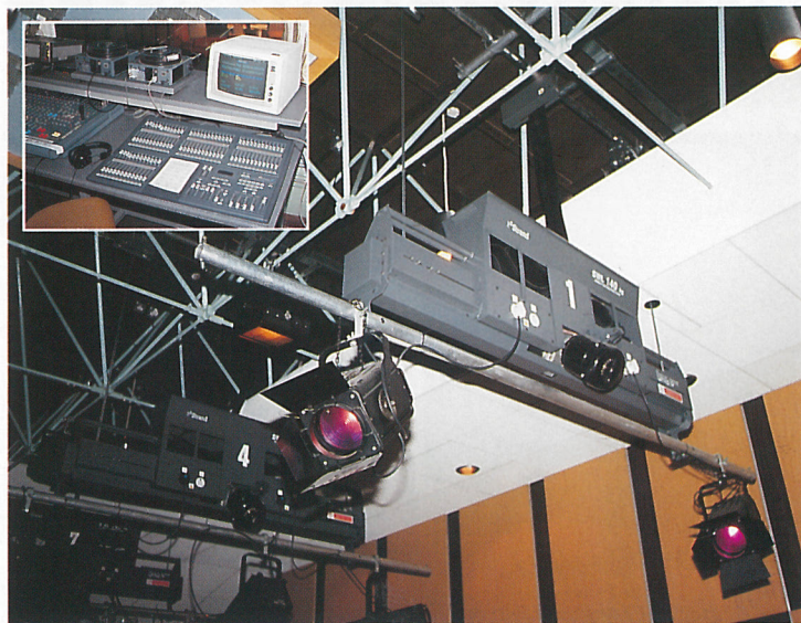
Control Room (inset) and Self-Climbing Hoist at Unilever Research.
