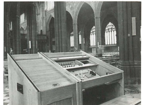
The Strand M24 Memory lighting system in Manchester Cathedral. The portable desk also houses the sound system controls.
