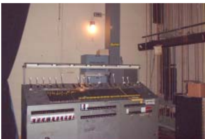
The original dimming system with its built in patch panel took up valuable wing space.
