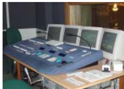
One of the two 550i consoles used in the theatre with its 4 monitors complete with Russian language displays. In the foreground are the Outlook architectural controls that were built into the main desk furniture.
