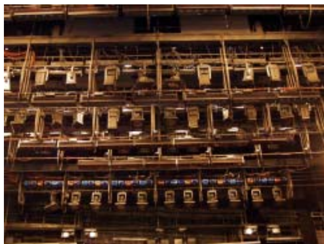
The first lighting bridges (sophits) at the new Bolshoi with its large rig of customer made Coda wash lights and Pirouette automated lights
