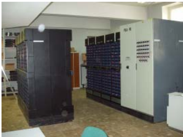
The main dimmer room with 14 SLD 96 dimmer racks
