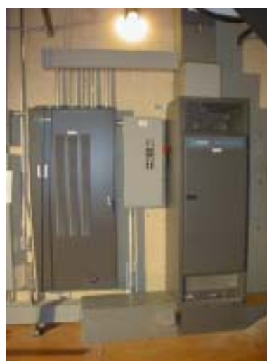
The new system provided more space back stage and increased capacity
